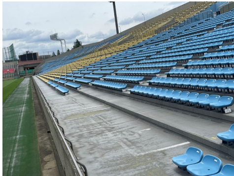
* Insufficient designated wheelchair spaces
